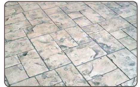
BEFORE: Old, faded, worn stamped concrete.
